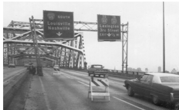
NOVEMBER 27, 1973 DAMAGED SIGN SUPPORT TRUSS ON KENNEDY BRIDGE APPROACH
