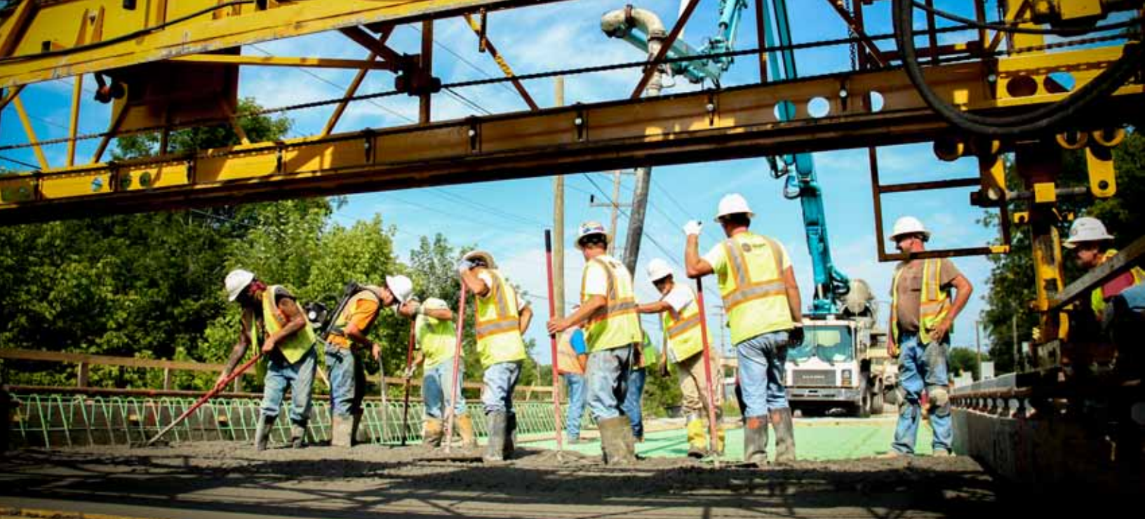
Researchers at the Center for Aging Infrastructure will cast sections of concrete, like those depicted here in the field, to evaluate the long-term performance of similar mixtures exposed to severe elements. This process can be used in model development and can be compared with field performance to better predict long-term performance. Photo provided.
