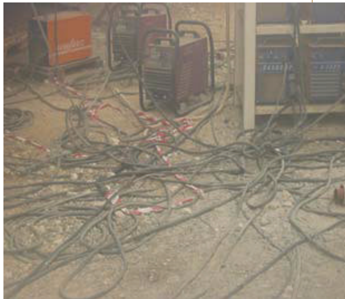
An example of poor housekeeping during a construction project.
