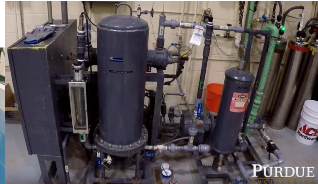
Coolant processing at PUR-1
