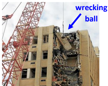
'Lady' – a crane equipped with a 4 ton wrecking ball – is used to demolish an old hospital in Norristown, PA.
