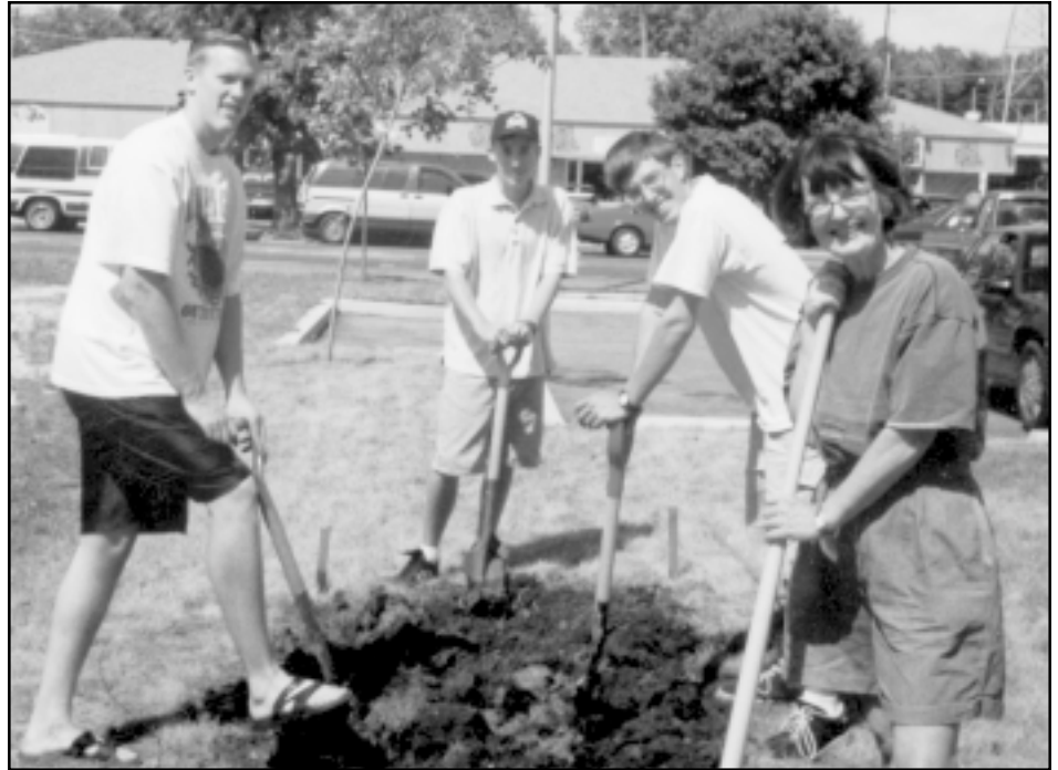
Lafayette Urban Ministry shelter volunteers Phil Thompson, Mark Anderson, Stephen Anderson, and Jo Johannsen prepare the ground for planting.
